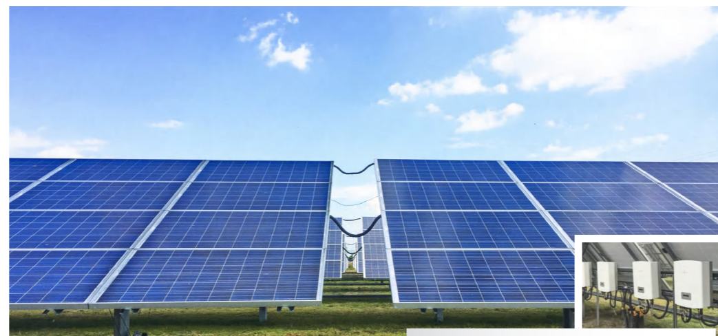
Mexico 20MW Solis-20K-HV
